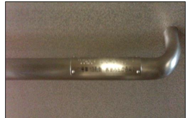
Braille plate on handrail
