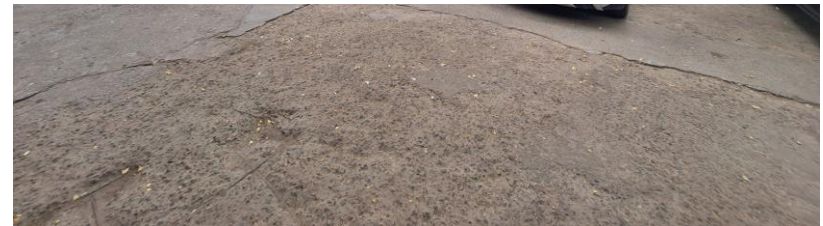
Damaged surface close to two wheeler parking space
